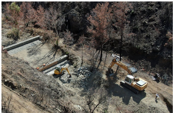
Retention works with gabions in channels affected by the Arakapas fire. Kostas Aristeidou, © courtesy of the Ministry of Agriculture, Rural Development and Environment of Cyprus.
