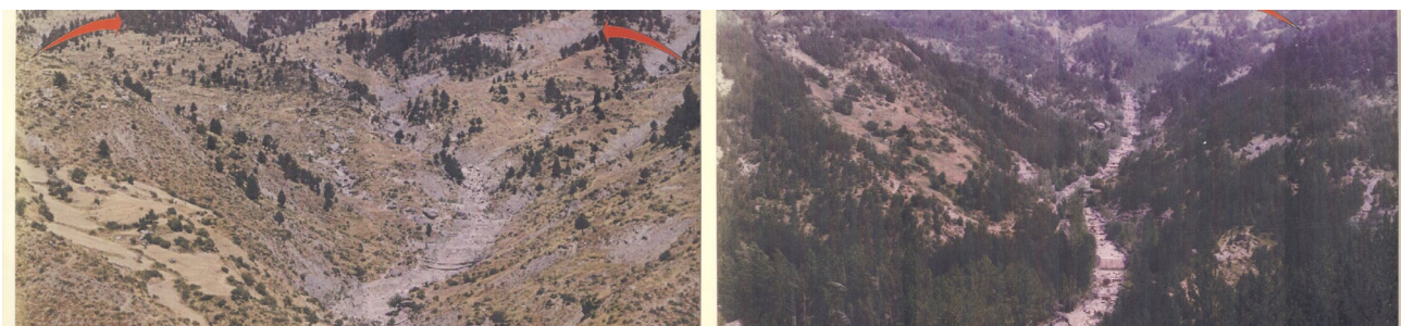
Evolution of the torrential correction works in the Metsovitikos ravine: from the initial state to the restored state. © courtesy of the General Secretariat for Forests and Natural Environment of Greece.
