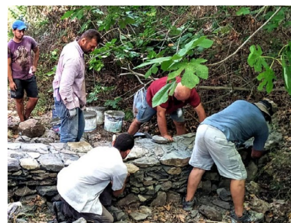
Construction of a micro-dam in the Karavas ravine (Kythira), thanks to the participation of neighbours from the community. @Zafeiriou © MedINA (Mediterranean Institute for Nature and Anthropos).
