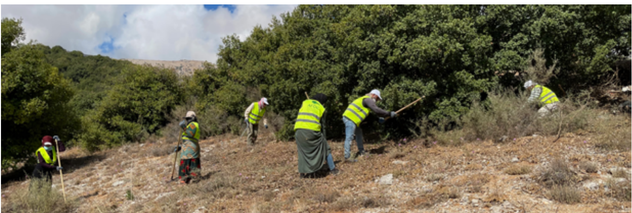
Work in progress of cleaning and clearing the forest cover in the West Beqaa district. Source: Ramy Sakr
