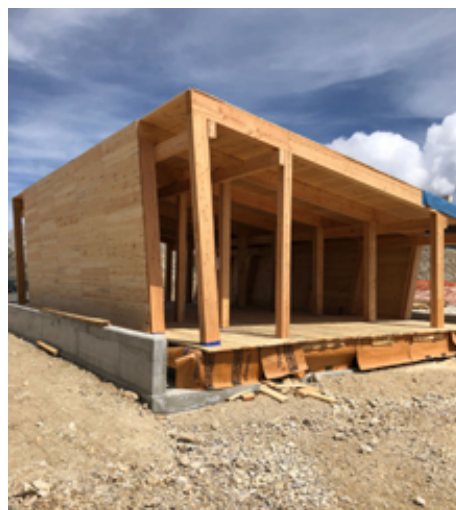
Construction of a mountain hut with pine timber from preventive interventions. Source: University of Turin
