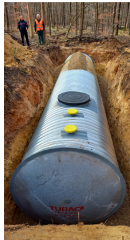
Installation of a buried 30 m 3 water tank. Source: ONF Fontainebleau territorial unit
